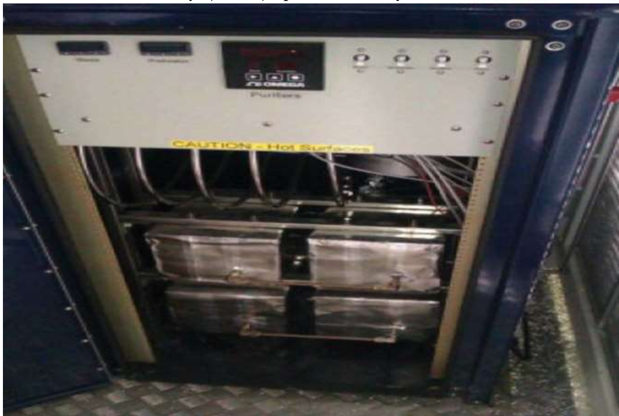
Picture 2. Dryer/heater/separator. Courtesy of Dr. A. Cruden.
